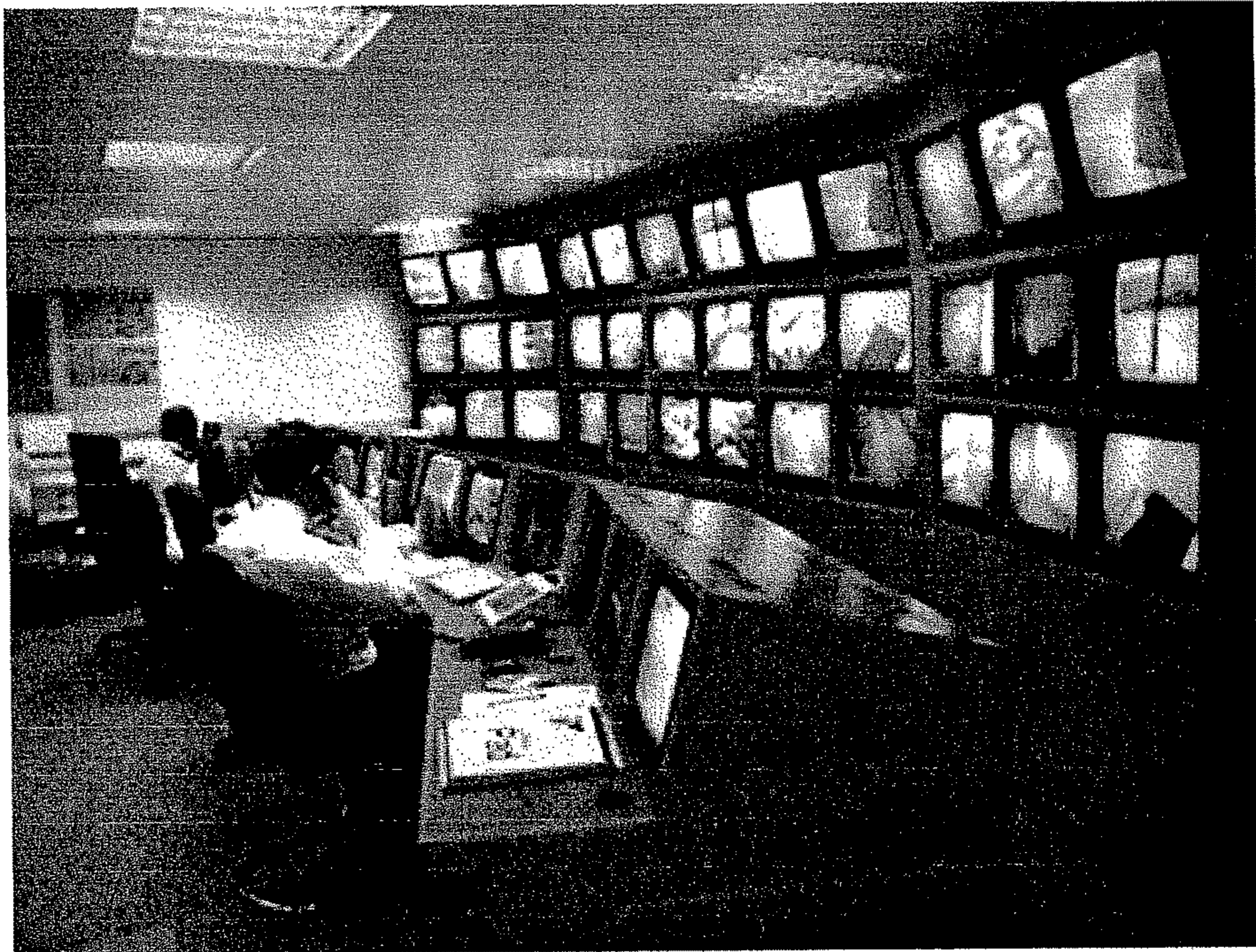
Figure 59 Typical Security Room
