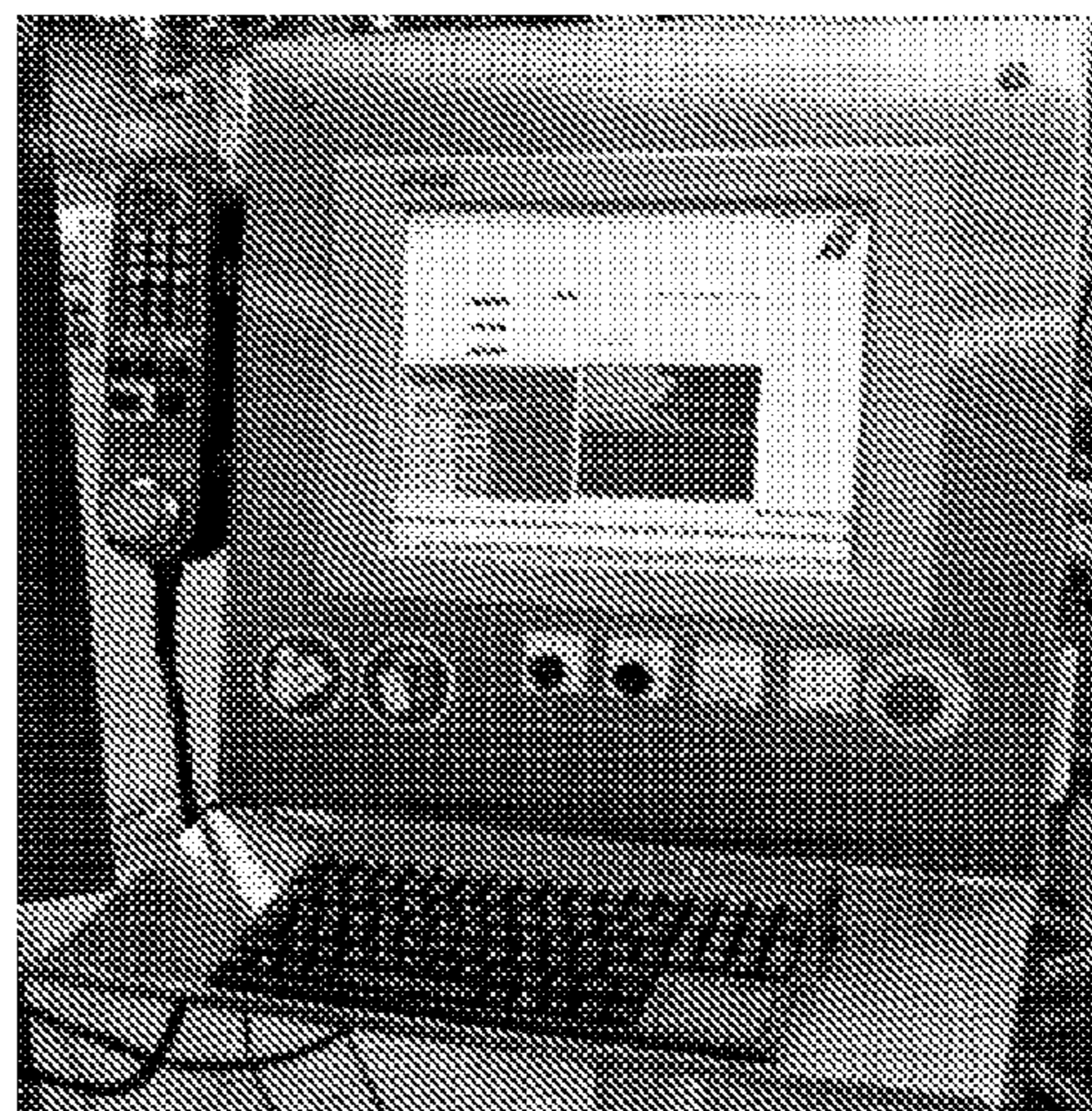
c) Control panel
