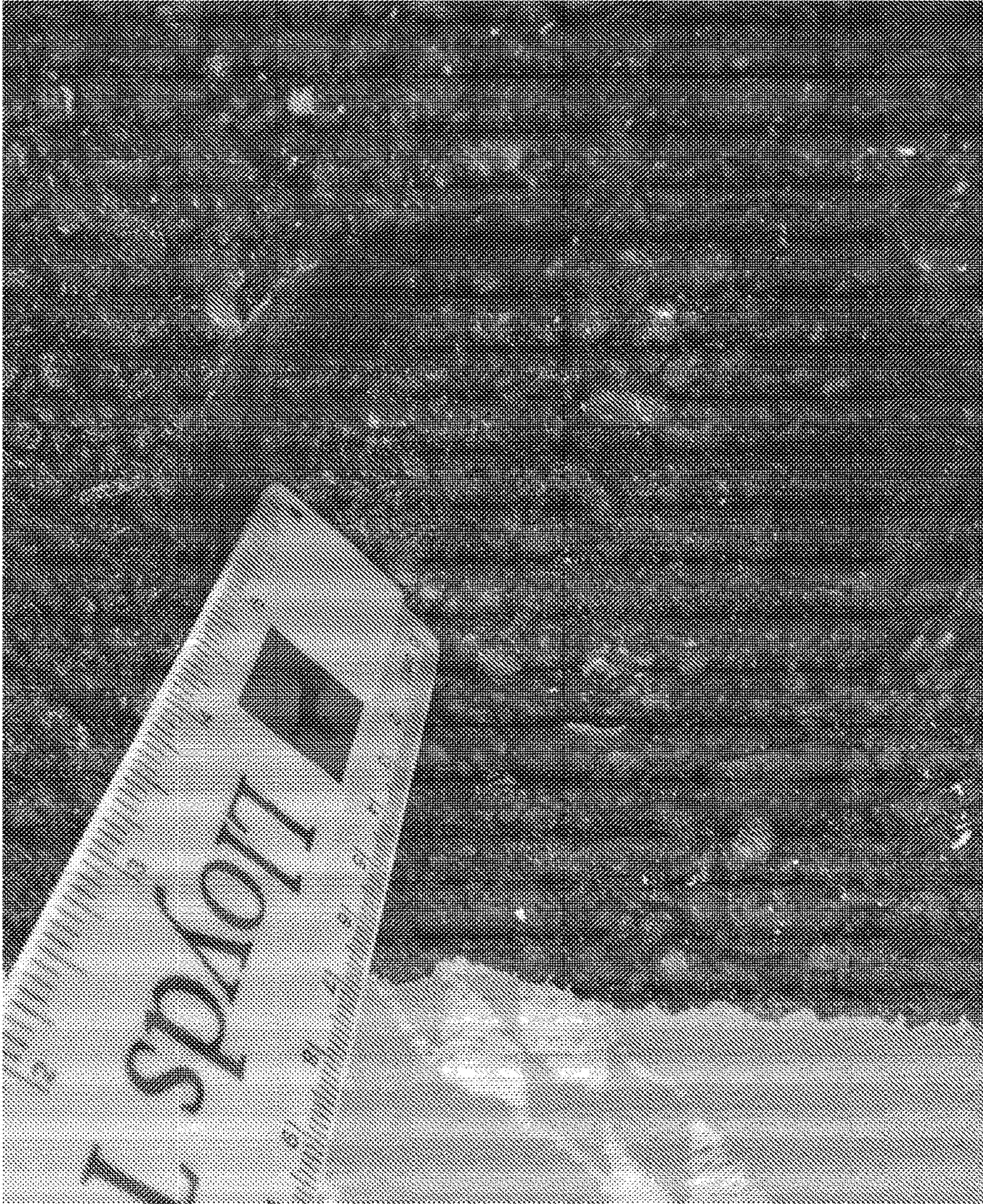
Asphalt Surface Before Repair
