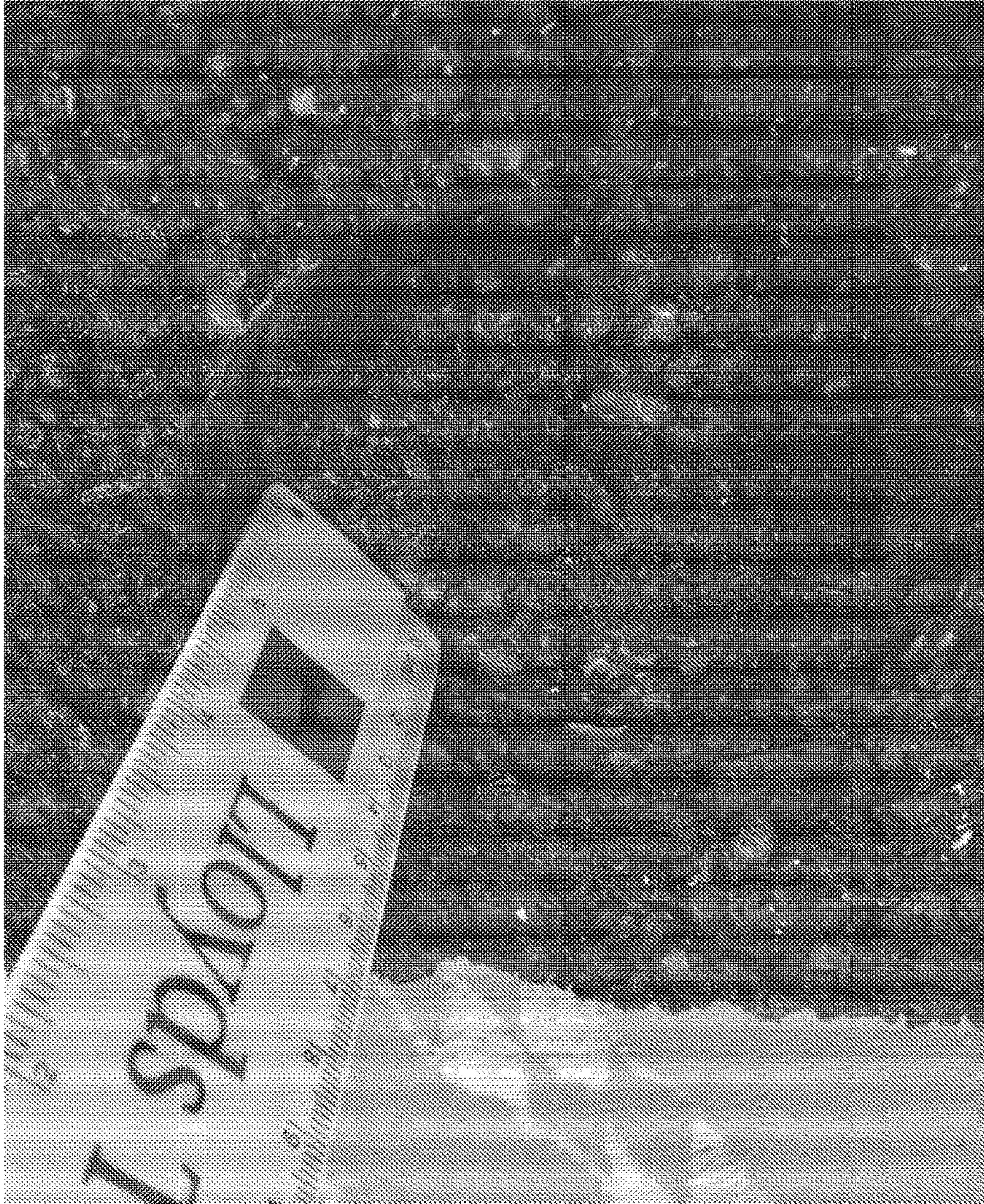
Asphalt Surface Before Repair
